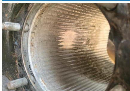
Trial fitting of CV driveshafts is important, especially on Mk2 cars which have this ribbing. The trial shows where the CV rubber clip catches and material must be removed with a flap wheel in a drill.
